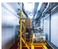
Local Equipment Room (LER)
